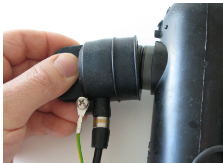
Fig. 4.11: Placing the test point adapter on the test point of the elbow connector
